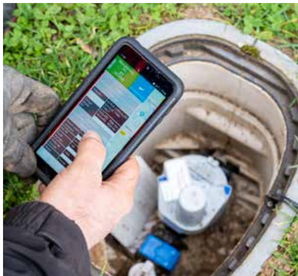
At operational level, our field technicians use digital tools every day to manage operations and optimize water supply network performance.
