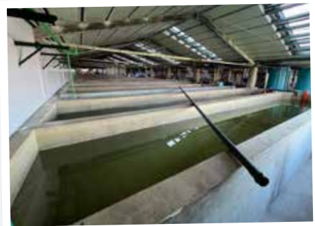
Pellestrina (Italy) – The VAL 600 AQUA system provides continuous purification of seawater for shellfish farms with minimal energy consumption.
